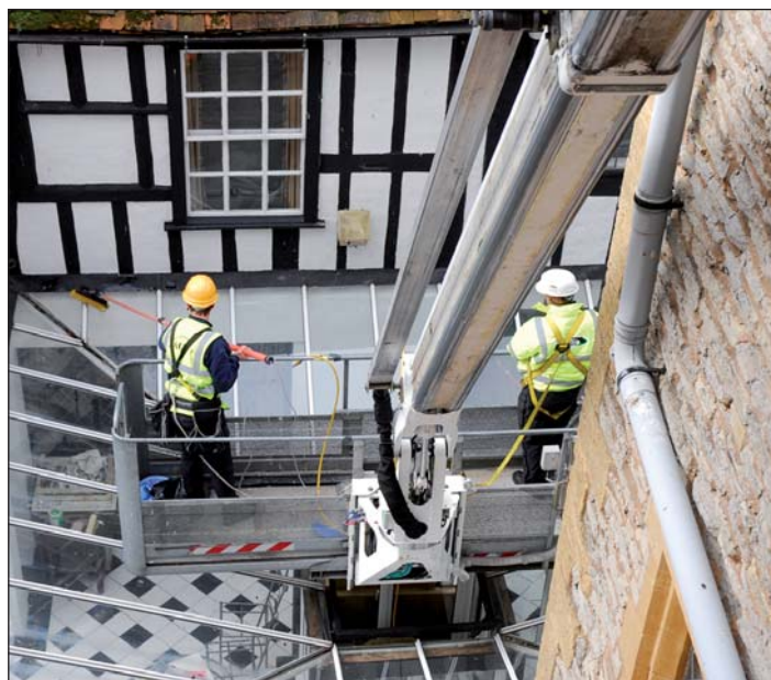
One of the trickiest areas to reach was an internal glazed-in courtyard - the Eagle's 17m jib and built-in pressure washer proved ideal.
