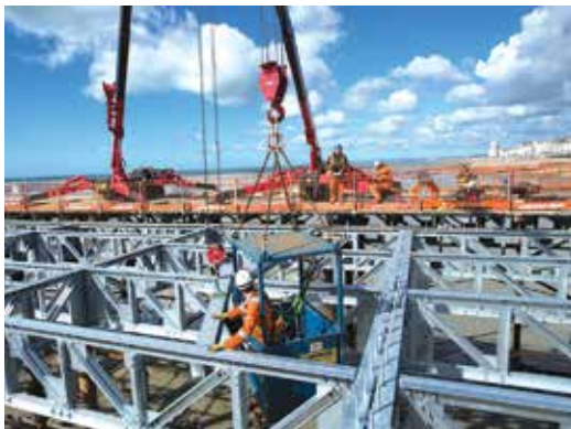
Unic 706 spider cranes from Coppard Plant have been helping replace 500 deck beams and 350 lattice girder beams.
