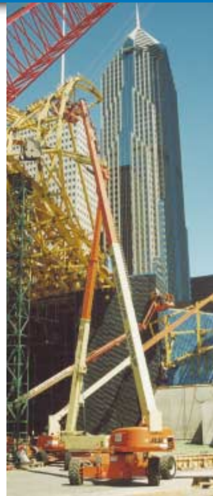
The job may require particular boom /jib configurations to reach the work
