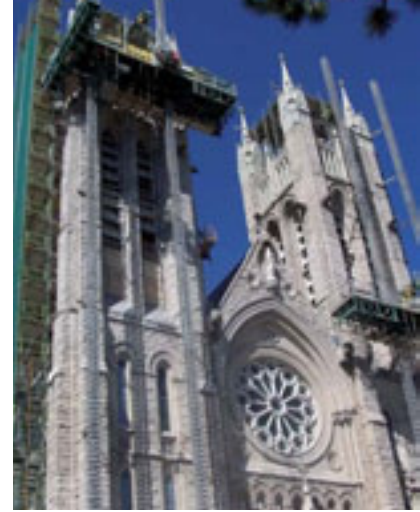
With Mastclimbers tourist attractions/city landmarks need not be covered in scaffold for years.
