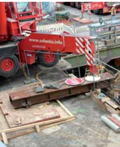
A well planned set up for a challenging lift over a new metro station. A precast concrete pad removes the slope, a large purpose-built wood mat and two reinforced I beams with clamps then spread the load onto a vertical beam.
