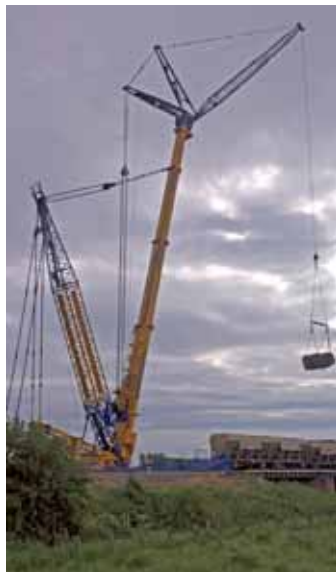
Due to the marshy fenland location and the extensive damage to the bridge, client Network Rail had to build a 1.3km temporary road so the crane could gain access to perform the lifts.
