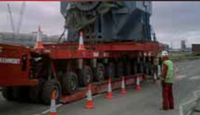
After the equipment was unloaded it was moved to its foundations using SPMT's.
