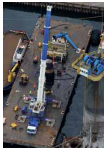
The Liebherr was placed on a barge to get in close to the thrusters.
