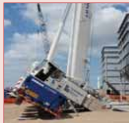
The owner of this crane was lucky, had he been properly trained in how to move a fully rigged crane?
