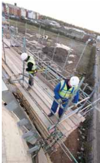
In spite of the obvious benefits that mast climbers offer façade scaffold is still the by far the most widely used access method for buildings.
