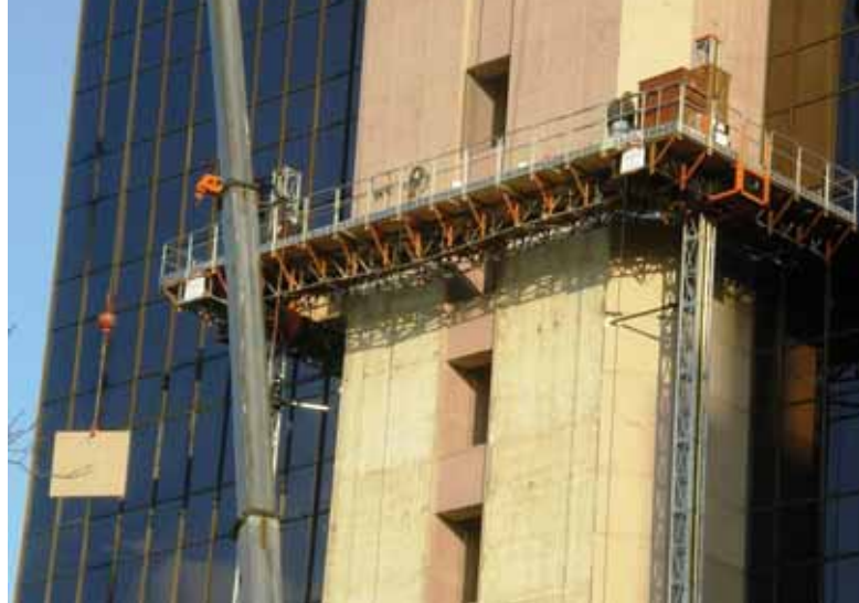
Working with a mobile crane over 200 stone cladding panels were removed in order to replace the steel supports and then refitted.
