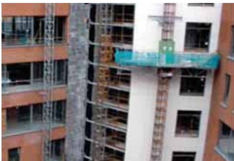
Mastclimbers are being used for construction and renovation of Belfast's Titanic Quarter currently one of the largest redevelopment projects in the British Isles.
