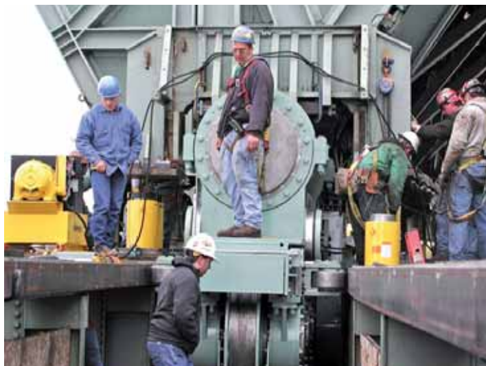
A new bogie in place. One wheel and two guide rollers are visible.
