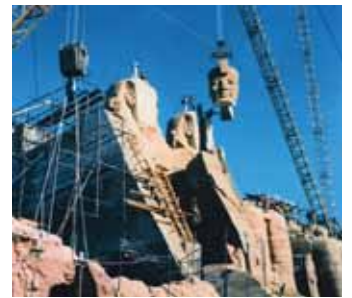
Wolff cranes were involved in the dismantling and reassembling of the two 13th century BC Ramses temples between 1963 and 1968
