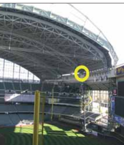
The roof is being lifted at the point circled in order to replace a bogie.
