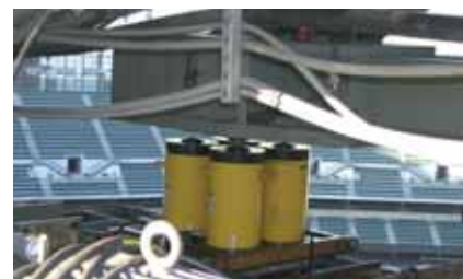
In this lift, the hydraulic jacks were arranged in a quad-cluster, fitted with spherical load caps and resting on a Teflon 'sandwich' to allow for lateral movement.
