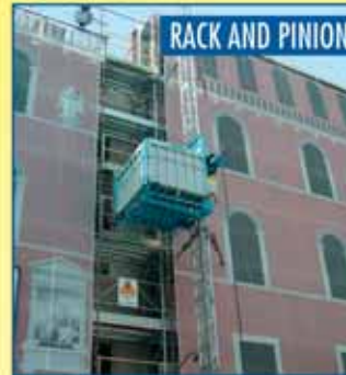
MAST WORKING PLATFORMS
