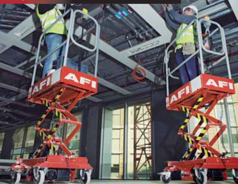
A total of 12 AFI Pop-Up machines are being hired by EA Electrical Limited to help install the fire prevention and alarm systems at the new Bankside 2/3 development on Southwark Street behind the Tate Modern in south east London.
