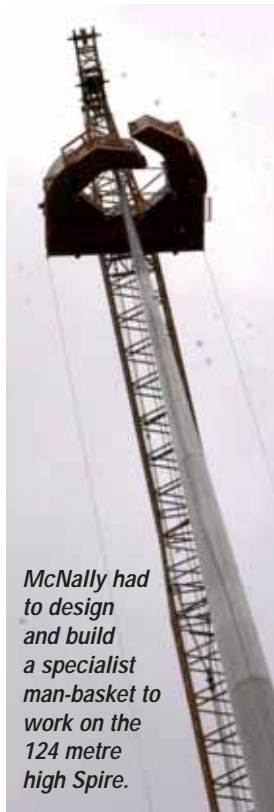
The 5 metre by 2 metre heavy steel frame basket used two hydraulically actuated 'wings' designed to envelope the changing diameter of the Spire.
