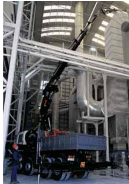
An unusual application for a truck mounted lorry loader. The largest can now lift to about 30 metres.
