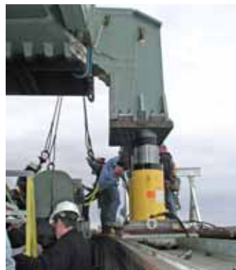
An old bogie being moved out. Two hydraulic Enerpac jacks are lifting against an add-on jacking bracket, as are another two jacks on the other side of the tracks.
