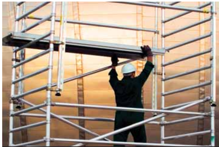
A temporary AGR, note that the guardrails are in place prior to the platform.
