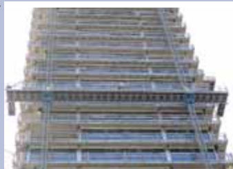
Two MBP02/150 mastclimbers were used, first on the long façades and then the ends. Platforms are 23 metres long with two metre wrap around cantilevers
