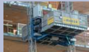
The MBC3500 transport platform offers a 3mx5m lift platform with 3,000kg capacity.
