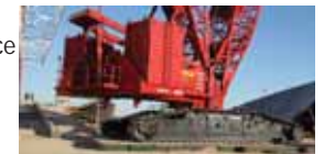
emtek mats providing a stable base allowing a 160t lift to be completed safely
