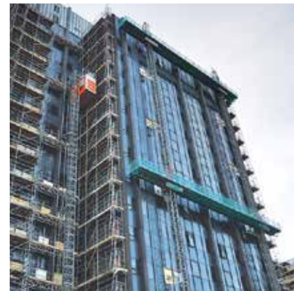
On the 17 storey Archway Tower which sits directly above the live Archway Underground Station Brogan is providing five, double-stacked mastclimbers mounted on heavy duty scaffold gantries.
