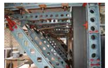
A cantilevered soldier bracket system fixed to the building façade - located above the station roof - supports the mastclimbers at four separate locations.
