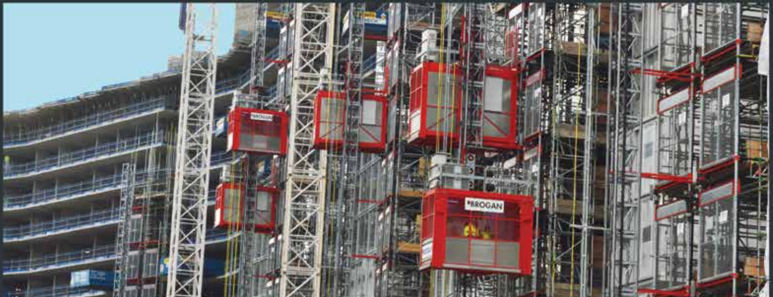
Twin Passenger/Goods Hoists Battersea Power Station
