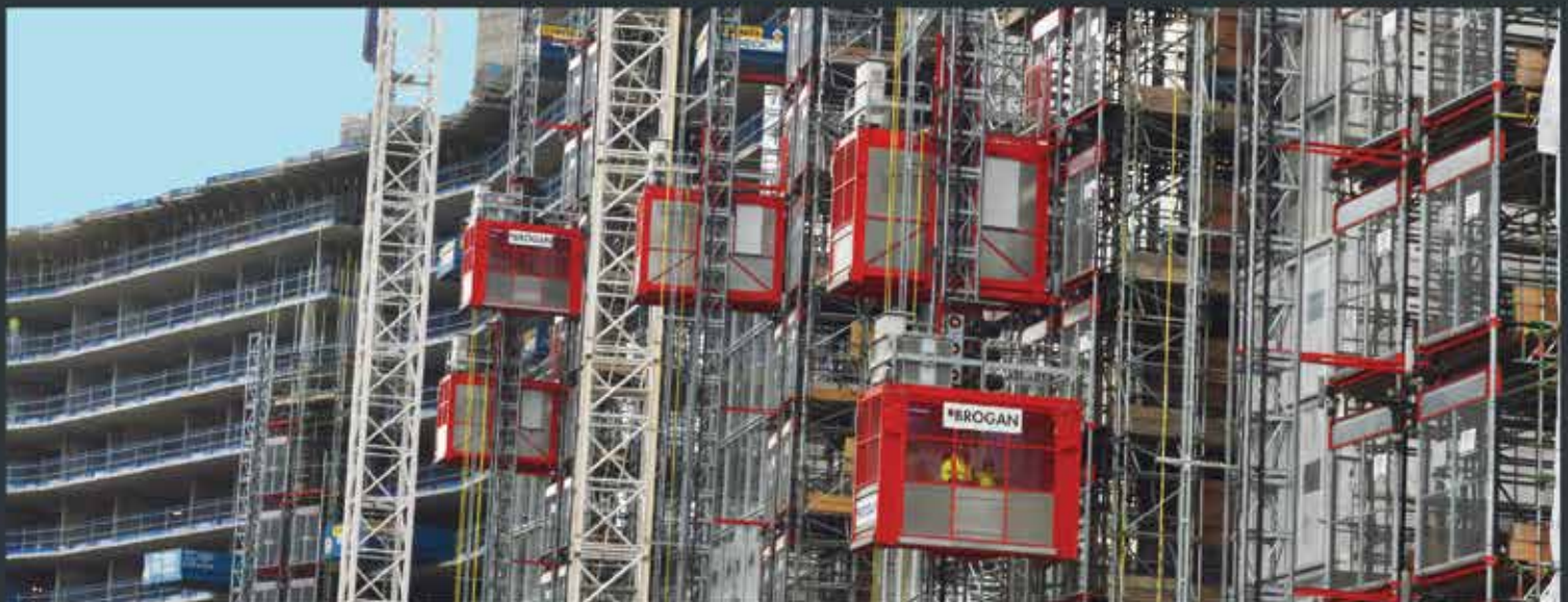
Twin Passenger/Goods Hoists Battersea Power Station
