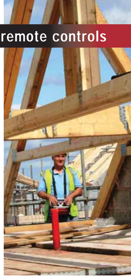
Operating with a remote allows the operator to often gain the very best view and be close to the placing of the load.
