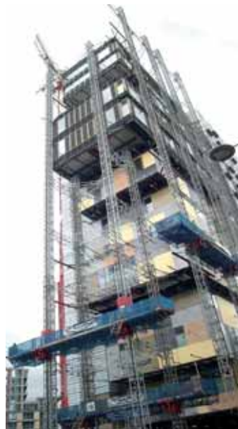
The North and South elevations required two twin mast platforms to be tied in back to back.
