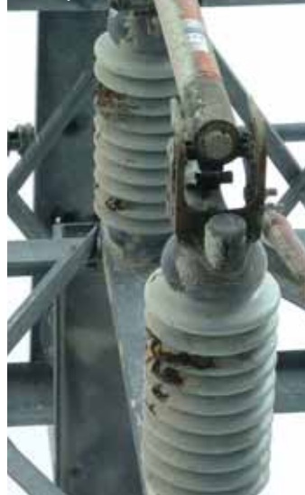
An insulator damaged from flash past
