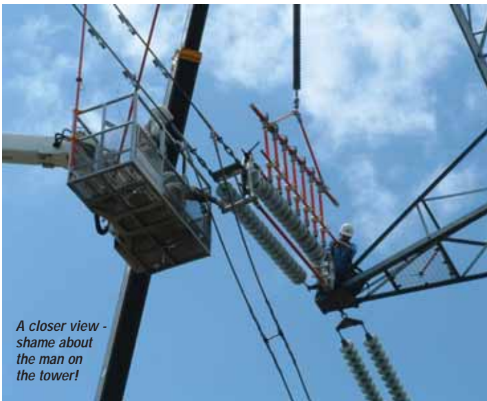
Here a crane with a hot stick lifting rod lifts an insulator
