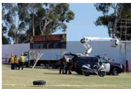
Daniel Pohl and Joshua Shetley were erecting a scaffold when Pohl came into contact with a power line.
