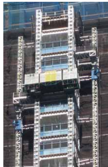
A Hydro Mobile mast climbing work platform is being used to construct the common tower as it grows with the building.
