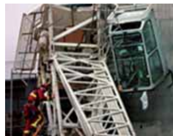
The crane driver was trapped in his cab for over an hour
