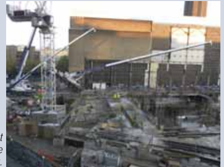
The crane tipped but came to rest on some steelwork.
