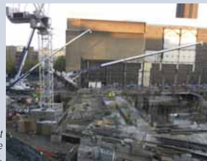
The crane tipped but came to rest on some steelwork.
