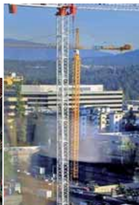
(Above) A picture taken prior to the collapse shows the crane (rear) was possibly up to a metre off vertical.
