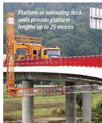
Although now aging, the Simon UB40 is still very popular for underbridge inspections
