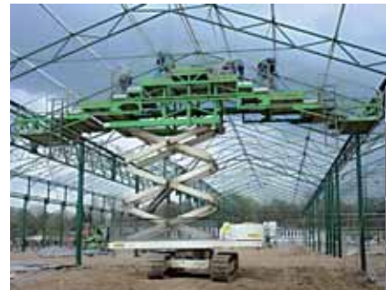
Some units are built with staged platforms to cope with pitched roofing
