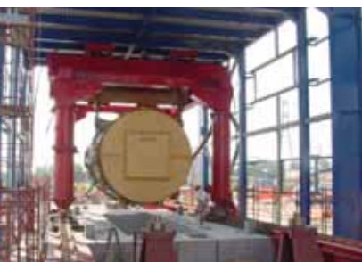
ALE's jacking system installs one of the gas turbines over the generator foundation at the power station in Turbigo, Italy
