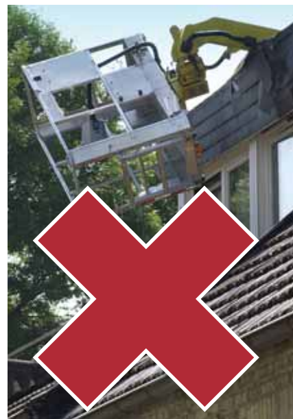
Two men died due to lack of a harness
