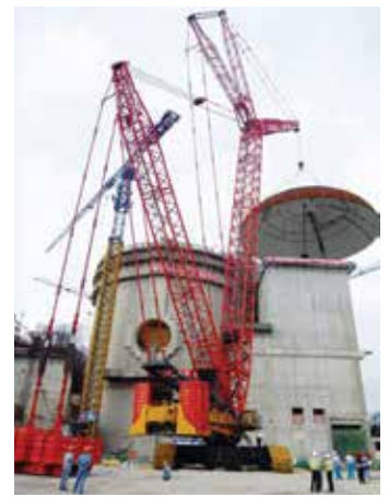
A Sany SCC9000 with 66m boom, 54m jib and 51m superlift radius to hoist the dome of No3 generating set which weighs 155t, is 11m high and 37m in diameter.
