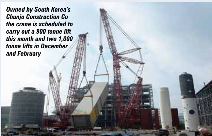
Manitowoc's largest crane the 2,300 tonne capacity 31000 crawler crane has completed its largest lift to date picking and carrying a 650 tonne cold box
