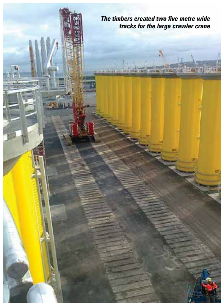
The 1,350 tonne crane is used to lift mono piles weighing up to 500 tonnes
