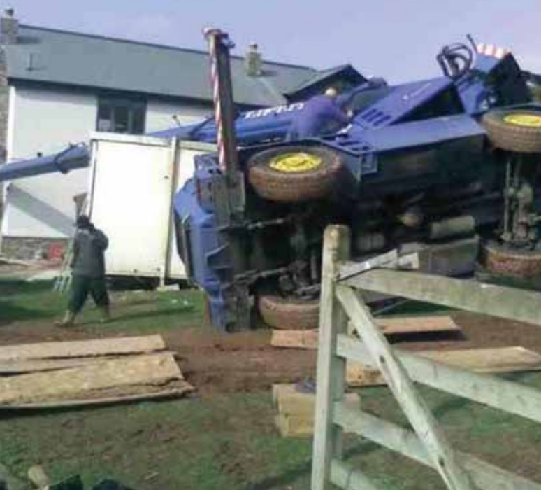
In this case the operator set up on hard frozen ground, but as the sun came out the ground softened and without a decent mat the outrigger jack sunk into the grass
