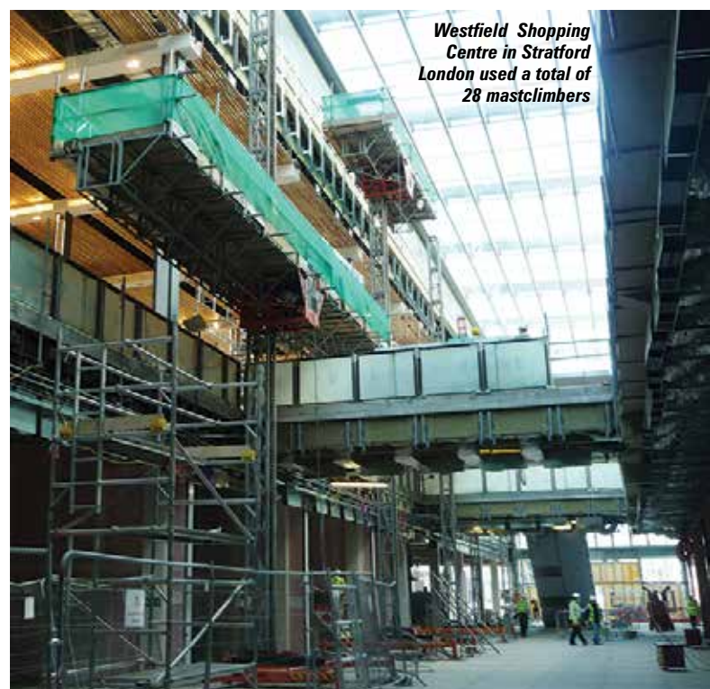
The gallows bracket allows the mastclimber to be set up avoiding low level obstructions
