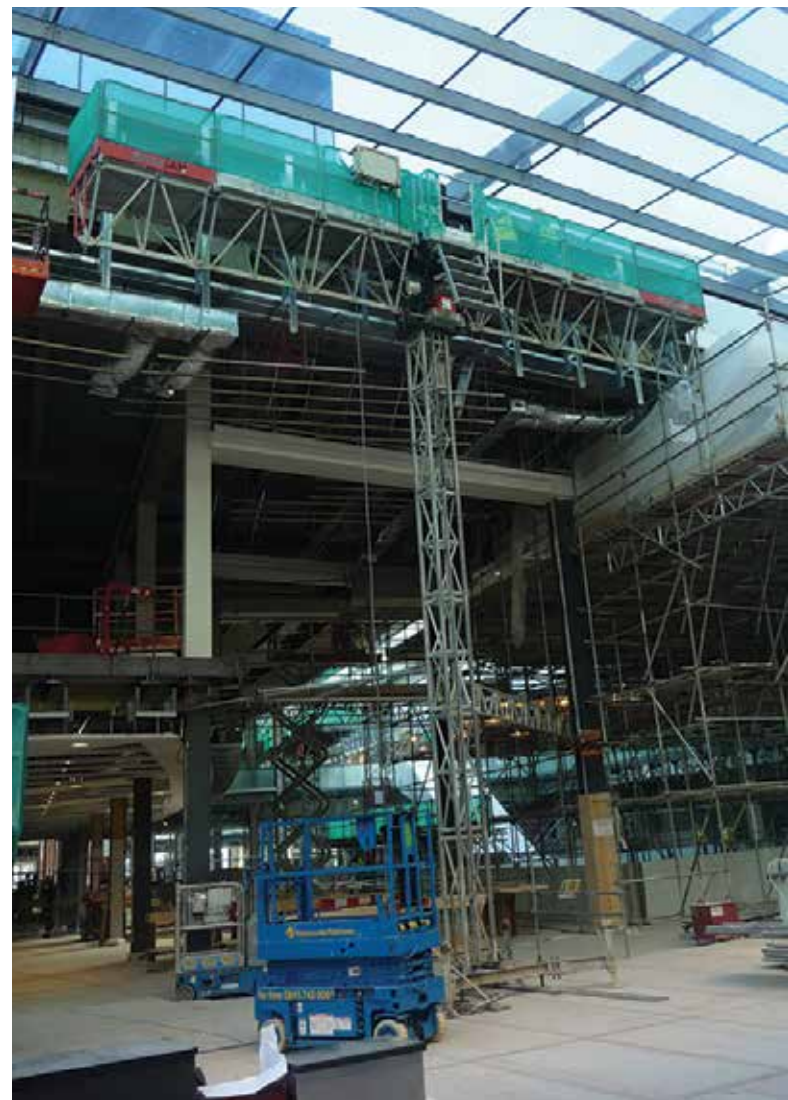
A 17m wide, 26m high mastclimber on the £311m Pinderfields Hospital development in Pontefract
