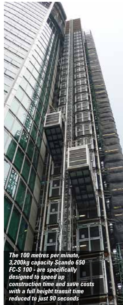
The hoist system installed at The Tower also incorporates a three by 4.6 metre 'Mammoth' hoist with a lift capacity of 5,500kg for the fast movement of larger materials
