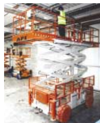
If you are using larger scissor lifts with black tyres and are concerned about your floor, insist that they are fitted with socks like these units, working on electrical installation at a new car parts manufacturing plant in Derbyshire.
