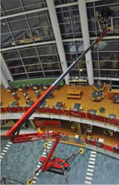
A Hinowa 26.12 tracked boom belonging to UK based MBS Access using Hi-Viz pads during cleaning the glazing in Central Milton Keynes shopping centre.
