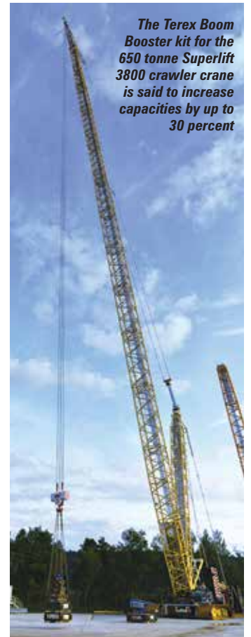
Bigge Crane and Rigging is using the first Manitowoc ML650 to erect a large wind farm in Minnesota, USA
