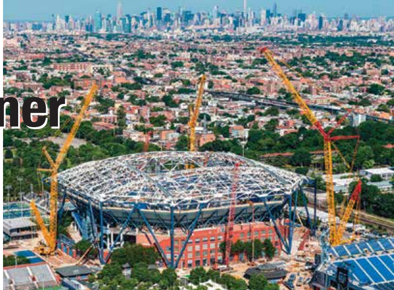
One LR 11000 and two LR 1600/2 cranes erect the steel structure for the roof on the Arthur Ashe Stadium in New York
