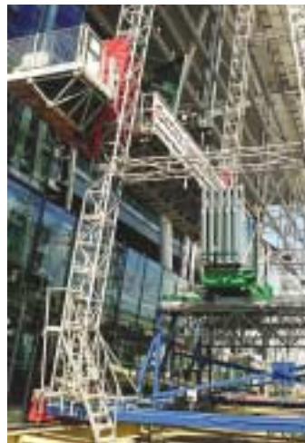
The pallets sat in motorised stillages.
