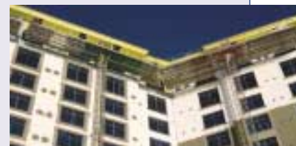
The 65 Scancrawlers provided wall to wall coverage with infill sections on most corners.
