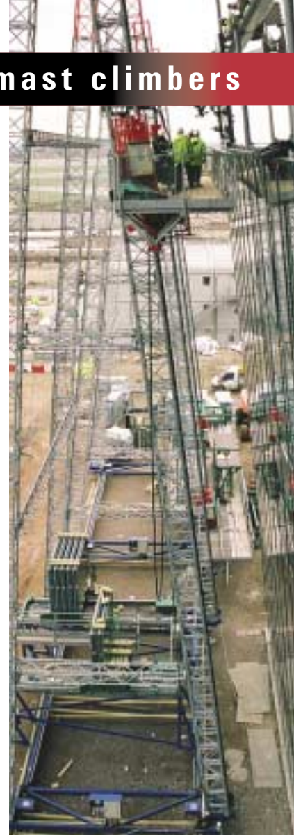
The solution to the access and lifting problem was solved with a twin mast A-Frame.
