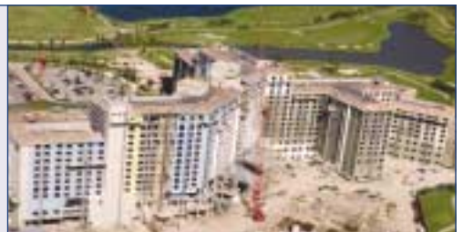
The Rosen Shingle creek is using 65 mast climbers on the exterior works.
