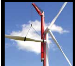
The Mammoet WTA 250 attaches to the base tower and installs the rest as it climbs its pre-installed track
