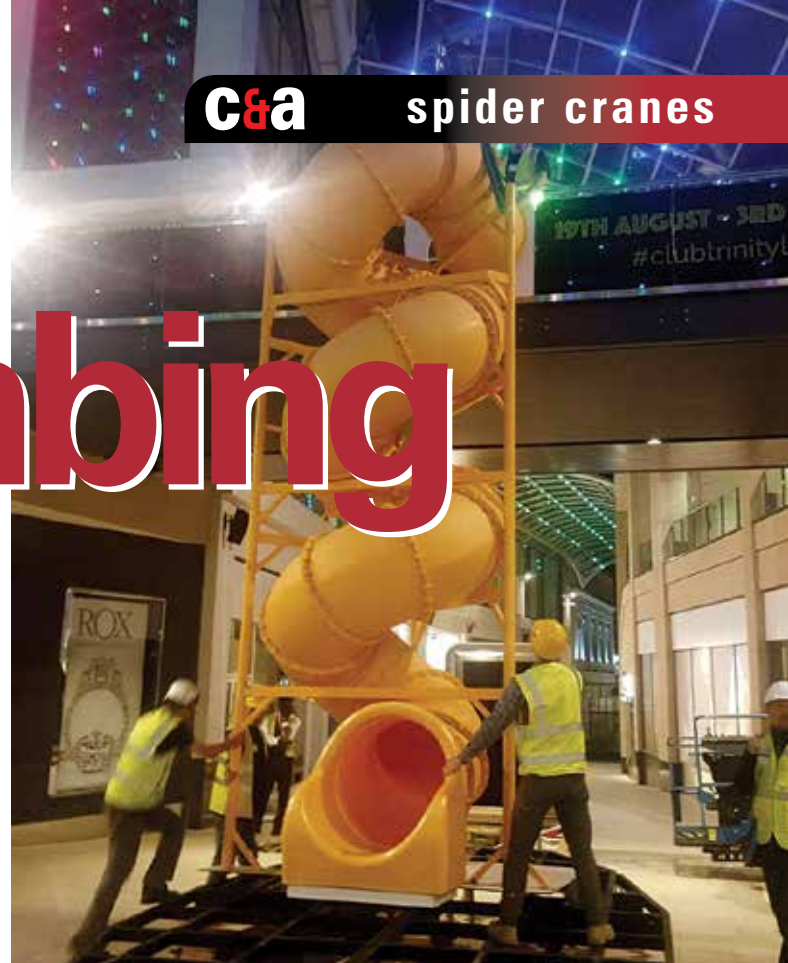
A Unic URW-506 mini spider crane installed a giant slide in the heart of the Trinity Shopping Centre in Leeds. The three tonne capacity, 16 metre lift height crane lifted the preassembled structure which weighed 1,000kg upright and manoeuvred it onto the pre-installed fixing points.
