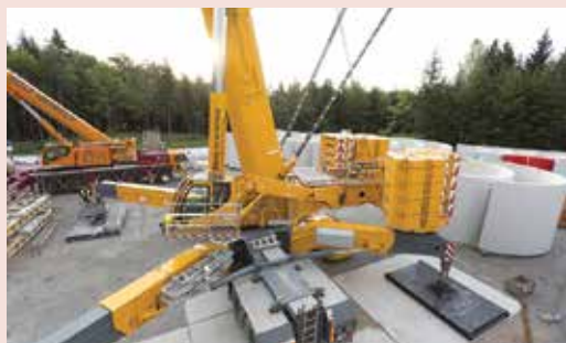
The maximum outrigger footprint of 13x13 metres provides the LTM 11200-9.1 the stability it needs. A 130 tonne Liebherr LTM 1130-5.1 is used as an auxiliary crane.
