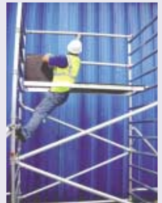
"Through the trap" one method of safely erecting a tower according to PASMA.
