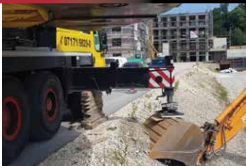
With insufficient space to set up, this All Terrain crane used the upturned bucket of an excavator. Not a recommended cribbing method!
