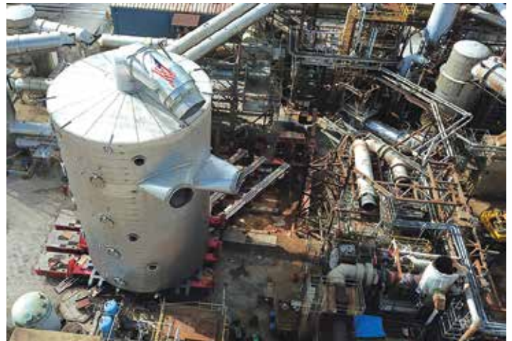
Mammoet designed a jack and slide system that could cradle both the old and new vessels at the foundations to elevate and slide them into place.
