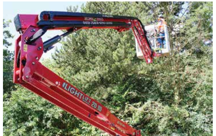
Dangerous as tree work is, it is far safer when carried out from an aerial work platform rather than actually climbing the tree
