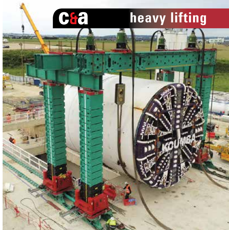
French heavy lift company Scales SAS has used an Enerpac JS-250 Jack-up gantry system to lift and lower Koumba - a 8.9m diameter, 11.4m long tunnel boring machine weighing 880 tonnes - in the latest phase of the Paris Metro extension project.
