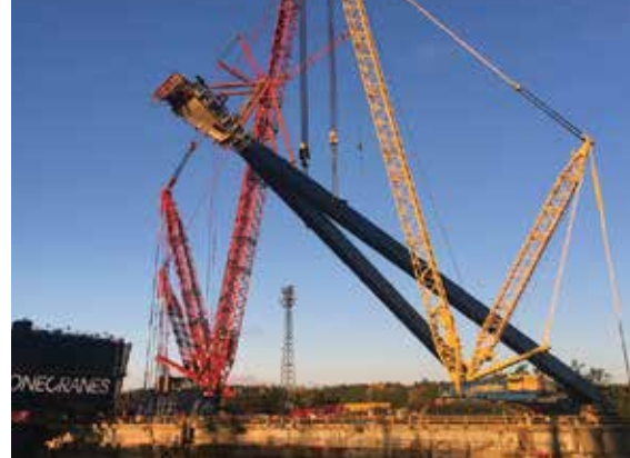
The Demag CC6800 and a Liebherr LR11000 erecting one of the gantry legs
