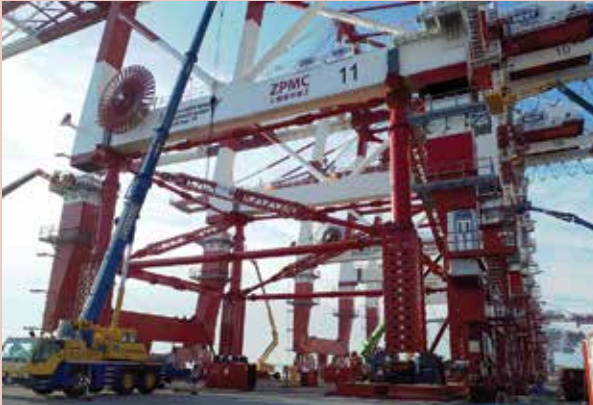
The Mega Jack 800 has 800 tonnes capacity in each of the four towers and performed the jacking in 12 stages.
