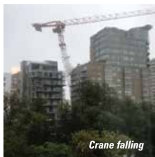
Halifax crane before it fell
