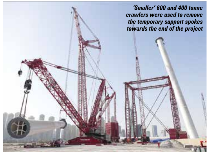
Mammoet's PTC 200-DS and Liebherr LR 130000 cranes installing the wheel's 1,900 tonne spindle
