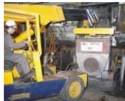
A Valla demonstrates a tough restricted headroom lift at Drax power station
