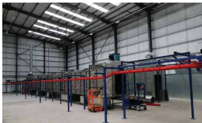
Installation of an all new state of the art paint booth is underway.
