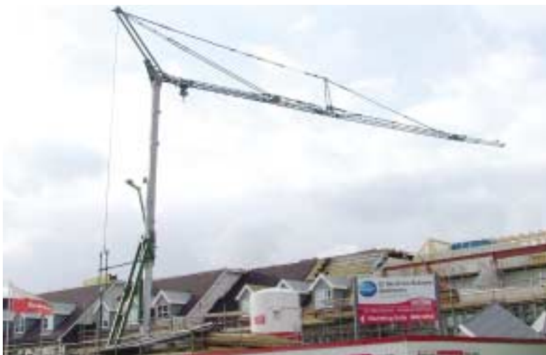
This three storey development is an ideal project for a self erecting tower crane.
