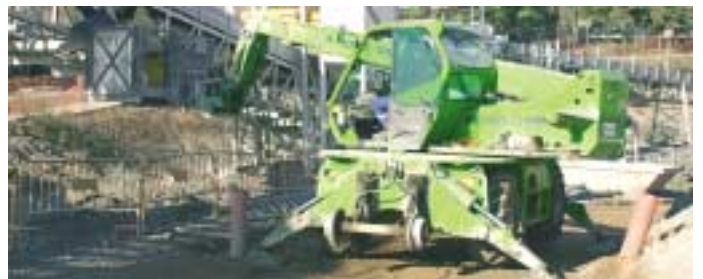
The units used on the Barcelona Metro include Tre Emme work platforms and road rail gear
