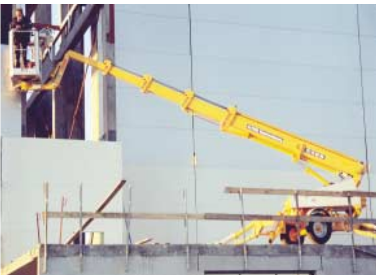
The Omme lift 2100E weighs just over two tonnes and reaches 21 metres, ideal for this job on an upper floor at the new Aarhus air terminal.
